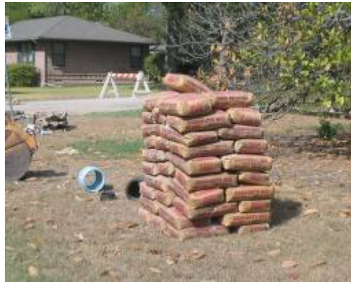
Figure 13: Concrete at the Job Site that was Unused for Thrust Blocks
